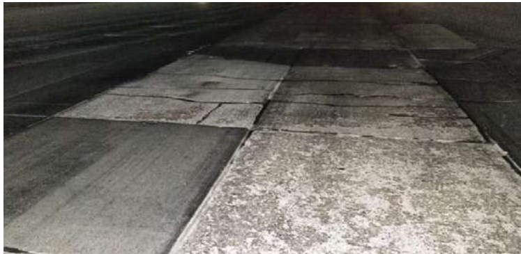
Figure 5. Defects on the runway.
