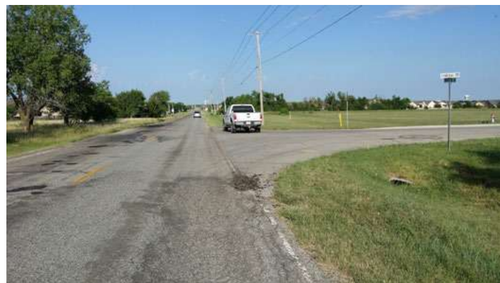
Figure 11. Pre-existing condition of Asphalt on East 45th Street, Wichita, KS
