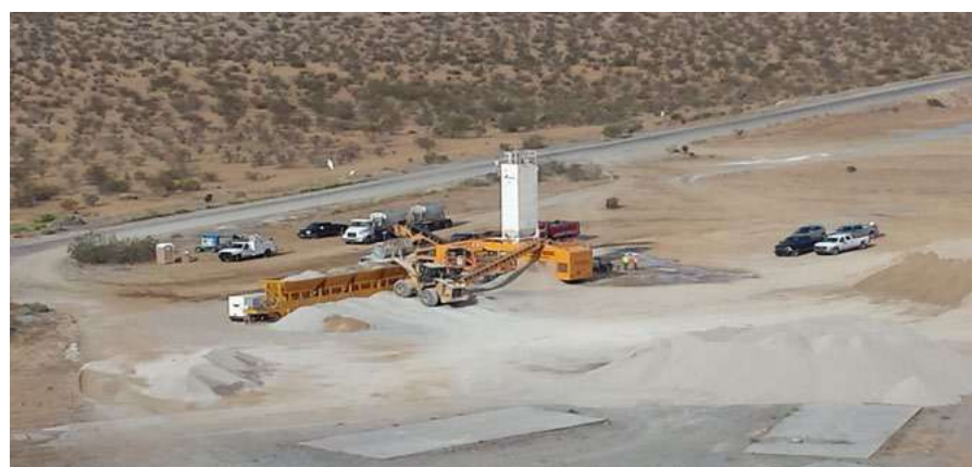
Figure 6. Pugmill Mixing Plant
